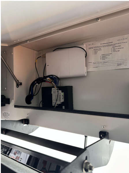
Mounted in Bus Cabinet
